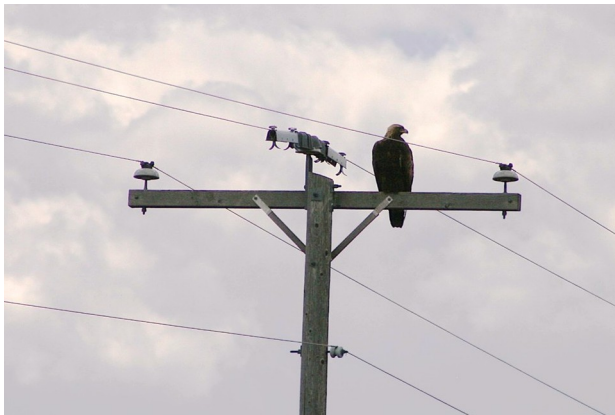
Golden Eagle perched on a power pole that has been retrofitted to be avian safe.
